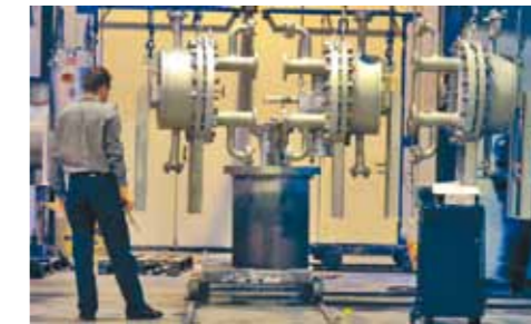
480 kW Raffinate Stripper Bottoms Cooler, PSHE 5HH-148/1/1
