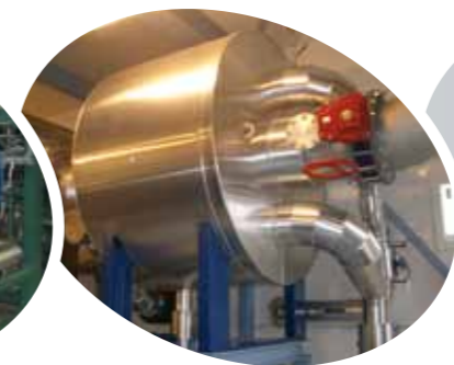
Gas drying Heat Exchanger in Landfill Gas Recovery system
