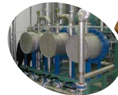
Industrial Heat Pump in Meat Processing Plant
