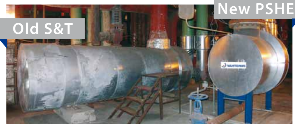
Successful replacement of S&T Heat exchanger in powerplant with significant space saving. 16MW PSHE 9HH-348/1/1 heating district heating water 64°C to 110°C using 0.9bar steam.
